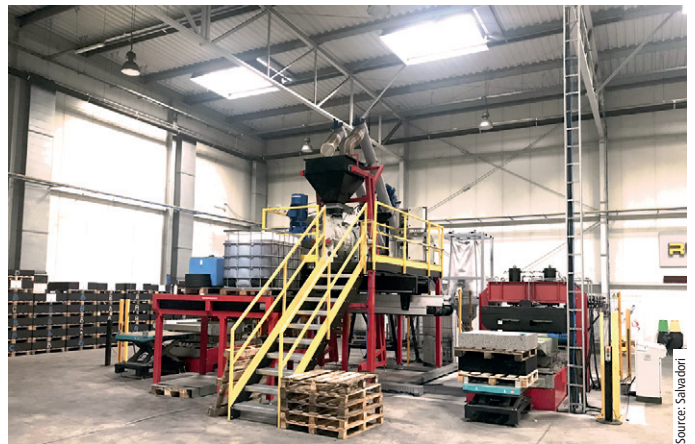
Fig. 5: It is also possible to produce rubber granulate blocks that can weigh up to 1 t, depending on their size. The maximum dimensions are up to 1,200 mm in width, 2,000 mm in length and 300 mm in height.
